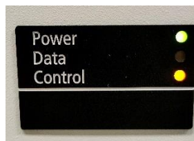
Power Light is On
