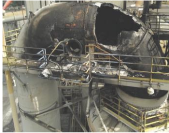
Fig. 2: After the fire
